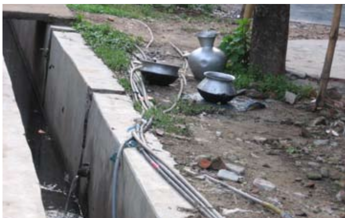
Illegal piped water system in Korail
